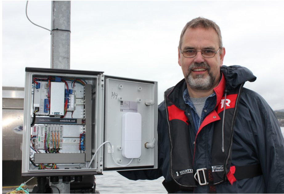
Founder and CEO of Embicon, Lars Magne Endresen stands next to an Embilink-A2 measurement station. Equipped with controllers from WAGO's PFC family, sensor data from a variety of manufacturers is collected and transmitted wirelessly, via cable or optical fiber to a server, which then stores the measured values in a database. Both real-time data and historical measured values can be graphically displayed on computers, smartphones and tablets.
