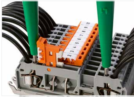
Testing with voltage tester.
