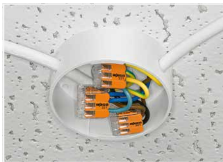
Lighting distribution in ceiling canopy
