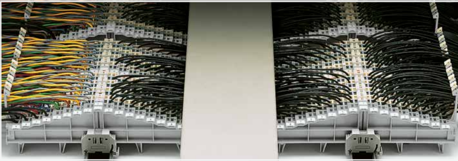
Example: Left: Main cables fed through locking clips on the field side Right: Control cables fed between locking clips Center: Wiring of both patching sides
