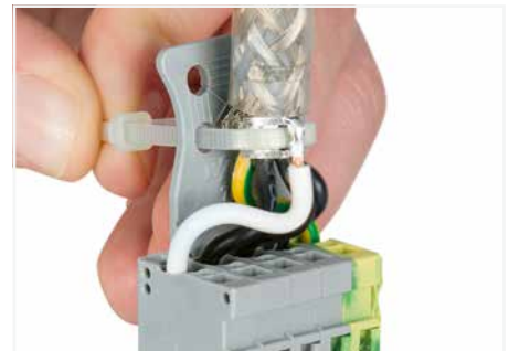
Secure both shield cable and shield termination to the strain relief plate using cable ties.
