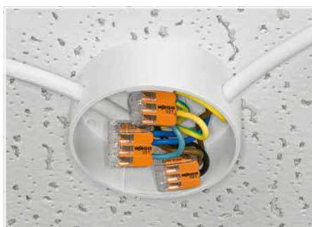
Lighting distribution in ceiling canopy
