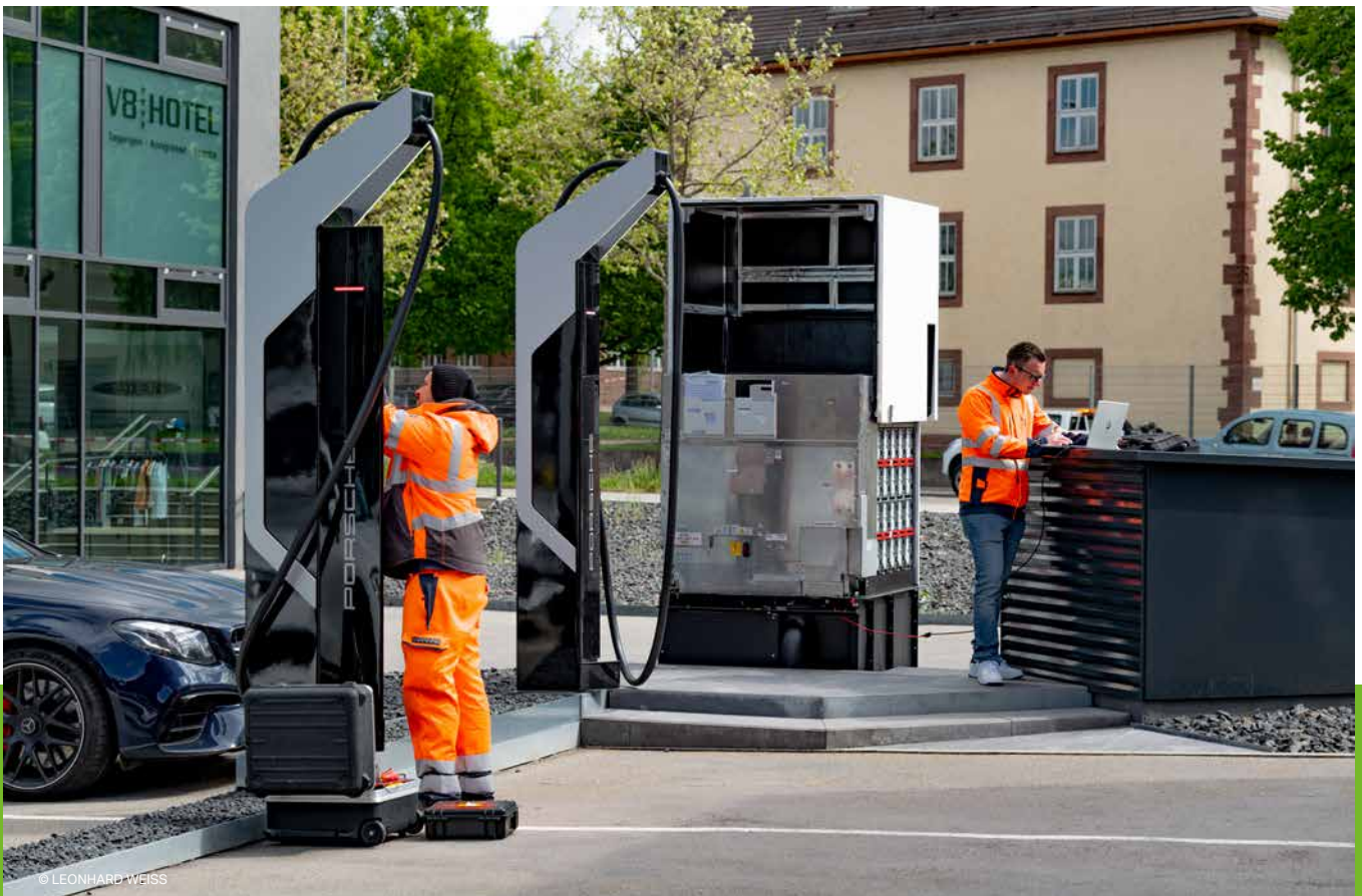
Before e-vehicles can charge at these DC charging columns, they must still be commissioned.
