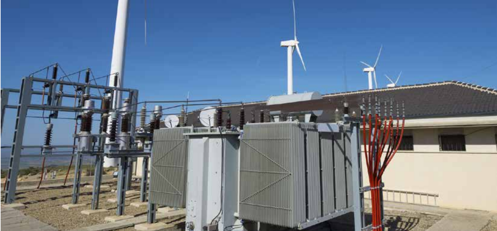
Substation at the foot of a wind farm
