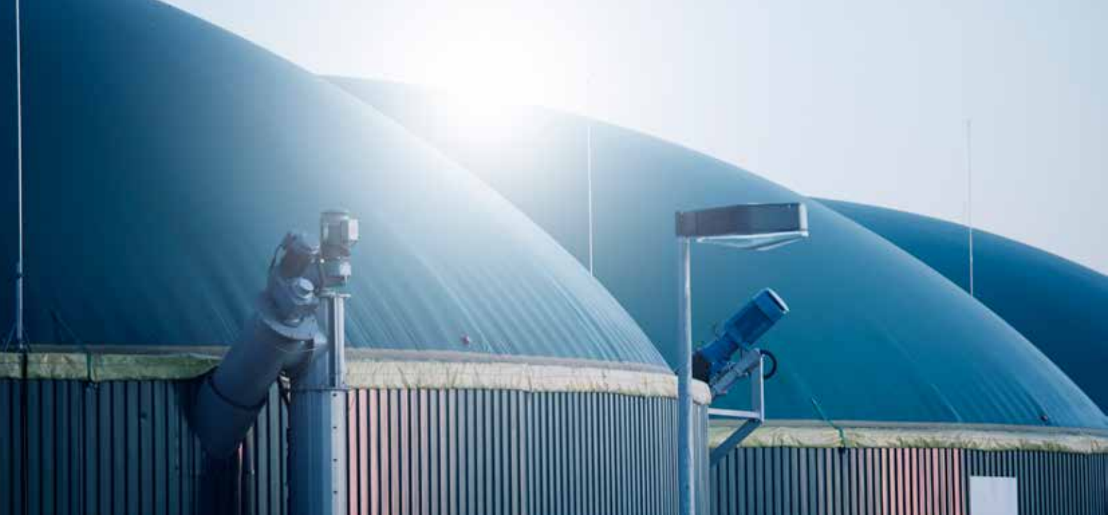
Biogas plant fermenters
