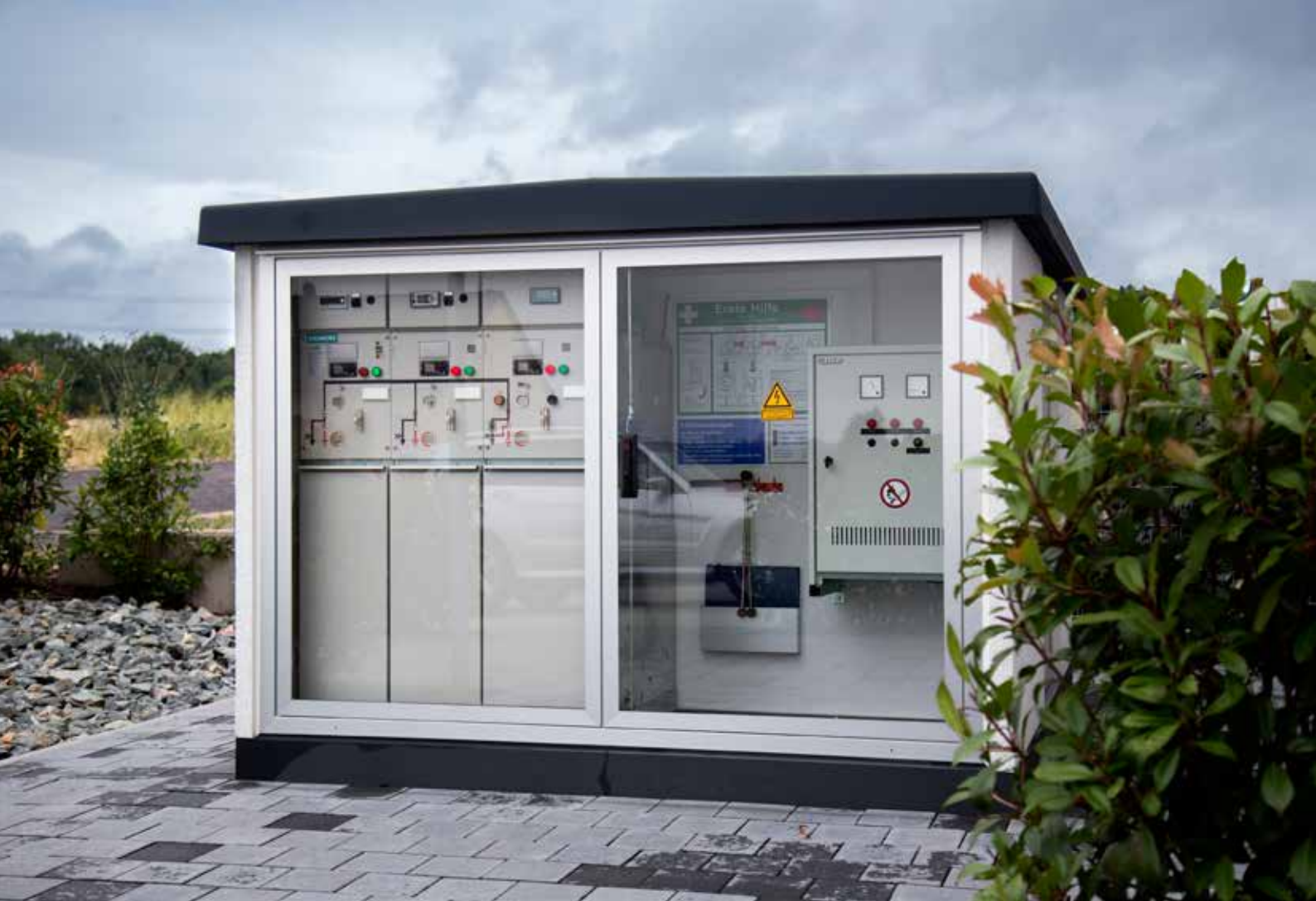
Intelligent distribution substation of Ingenieurbüro Pfeffer
