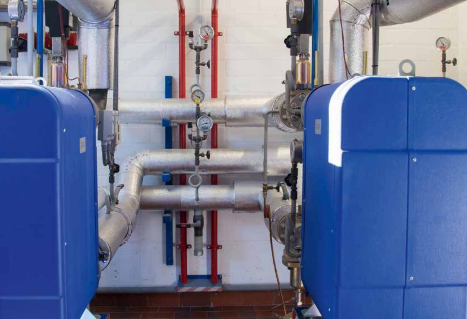
Flensburg municipal heat transfer station
