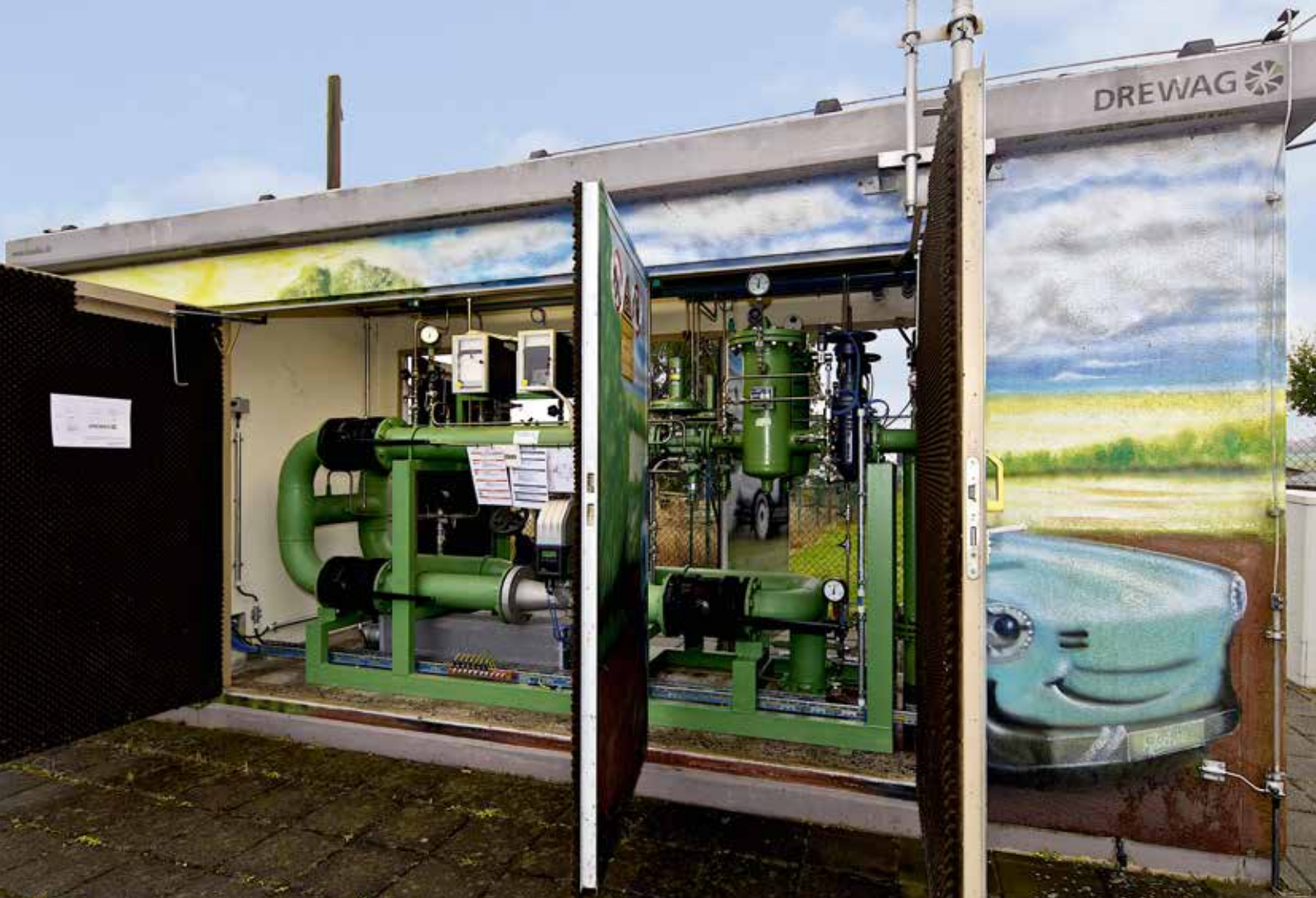
DREWAG gas pressure regulating station
