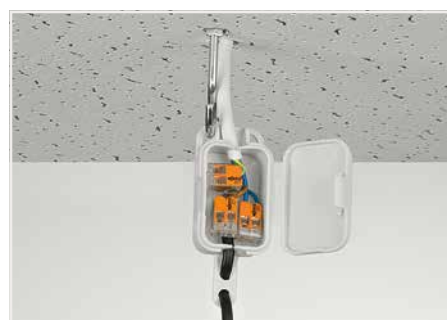
Pendant light connection in a suspended ceiling
