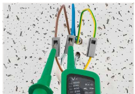
Testing via separate test ports.
