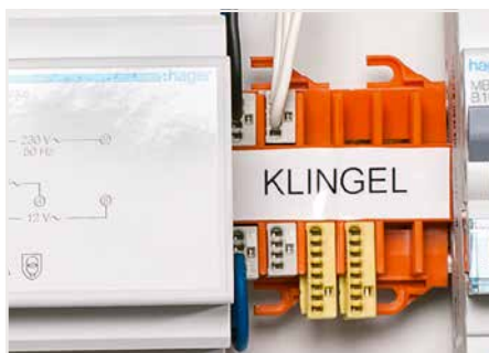
DIN-35 rail-mount application (residential door bell)
