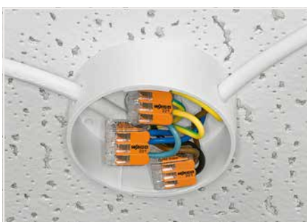
Lighting distribution in a ceiling canopy
